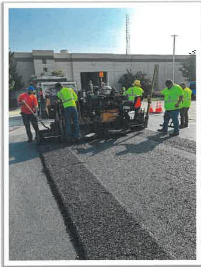
Crews are removing the wearing surface of the Mill Road viaduct over I290. The pavement was then patched with hot mix asphalt.
