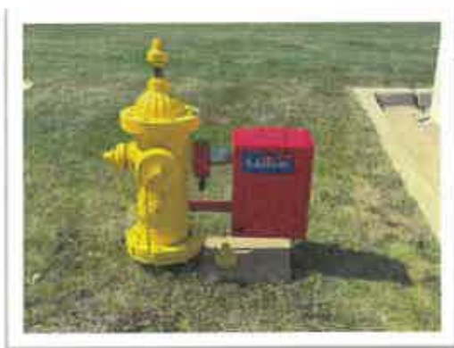
Automatic Hydrant Flusher
