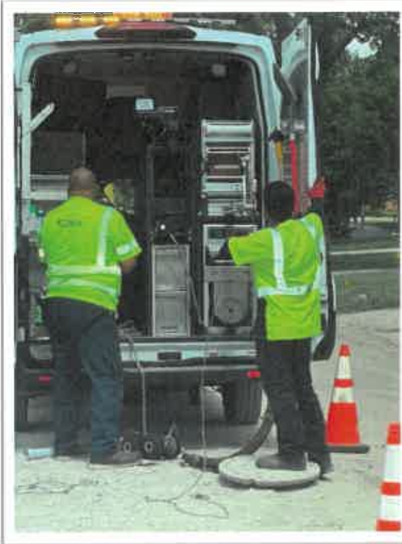
The Sewer Division is televising in the Home Addition area to help locate deficiencies.
